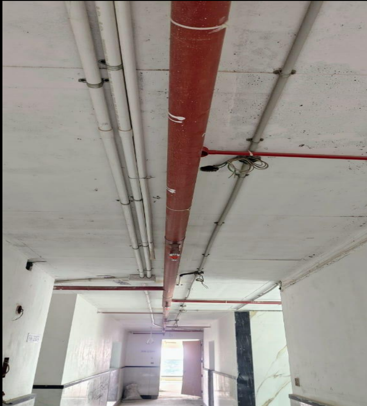
36. Tower B 45 th floor Corridor ceiling pressure pipe line work in progress
