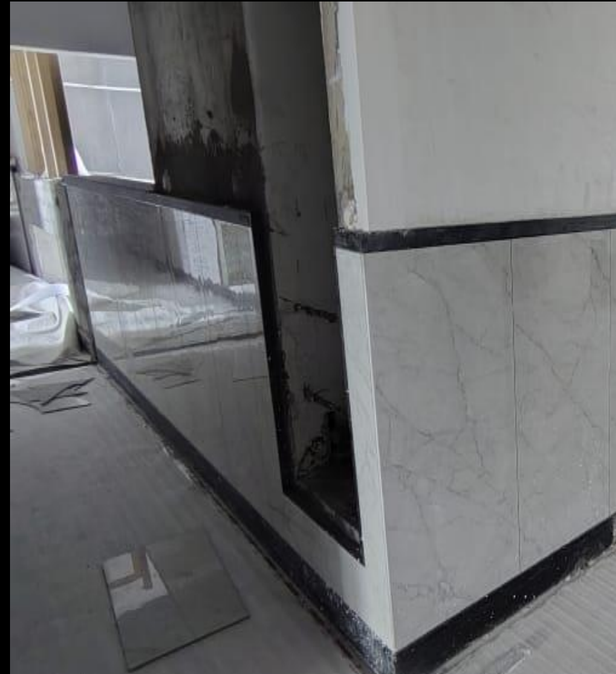
37. Tower B 45 th floor Flat entry main door side - wall dado work in progress
